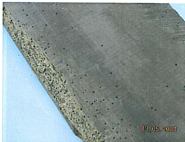
Anobium Borer Timber Damage
