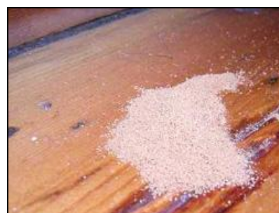
Anobium borer damage to floorboards
