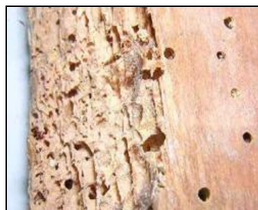
Anobium borer damage
