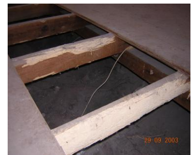
Lyctus borer damage to floor joist.
