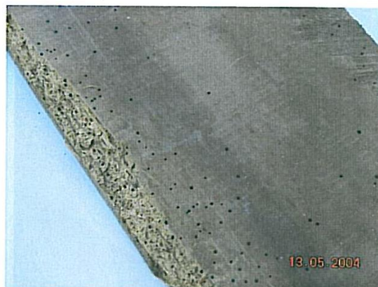
Anobium Borer Timber Damage
